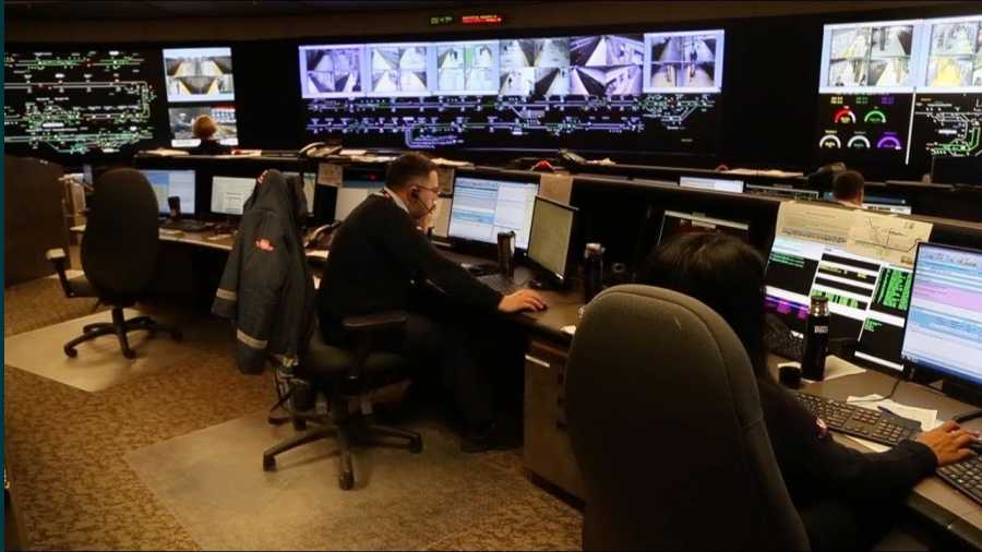
Communications Operations – Underground C2 Operations
